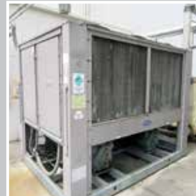
CARRIER 30GTN070 Chiller
