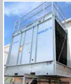
MARLEY Cooling Tower
