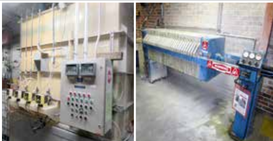
Waste Water Treatment Plant
