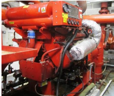
Detroit Diesel Fire Engine pumps (3-off)
