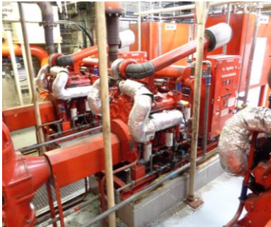
Detroit Diesel Fire Engine pumps (3-off)
