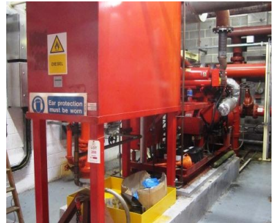
Detroit Diesel Fire Engine pumps (3-off)
