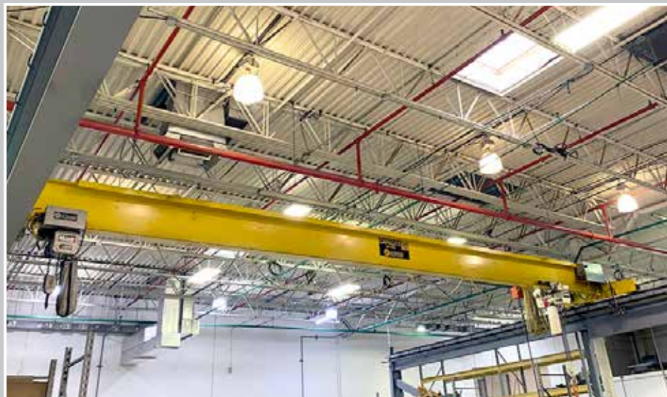
ALPHA 2000, 10-Ton Overhead Bridge Crane
