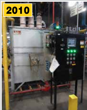
SURFACE COMBUSTION Generator
