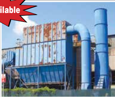
View of Dust Collector
